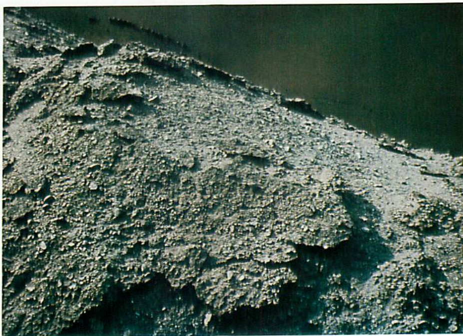
PLATE NO. 2: INCOMPLETE COVERAGE OF SLOPES
