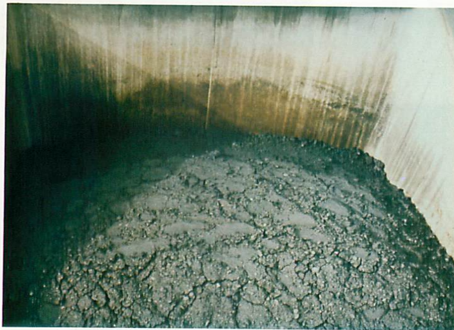
PLATE NO. 20: LIMITED CRUST FAILURE OF SLOPED AREA IN CAR IN PLATE 19
